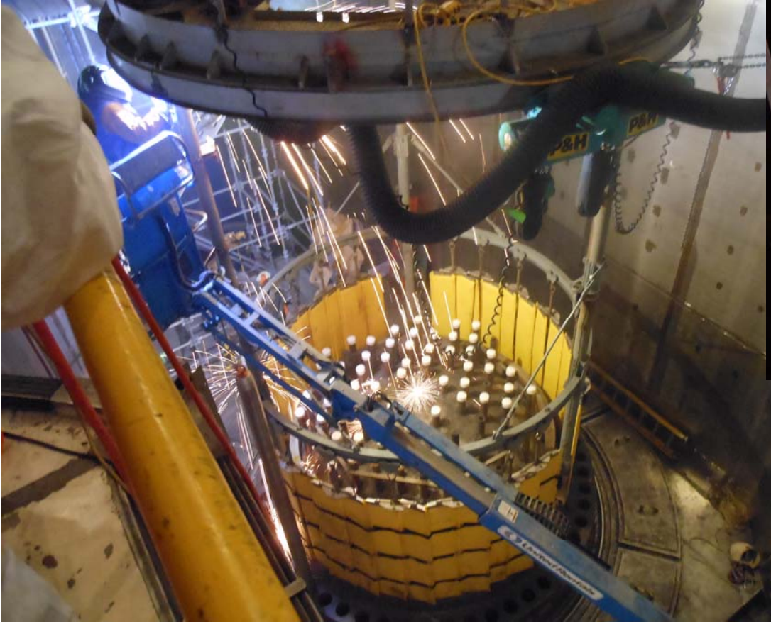
Reactor Head Inside Cavity
