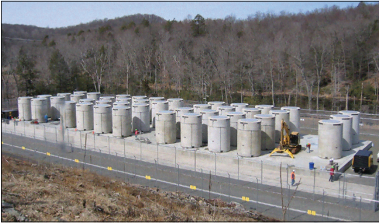
Independent Spent Fuel Storage Installation (ISFSI) Zion Station's ISFSI will be similar to the one pictured here in Connecticut.
