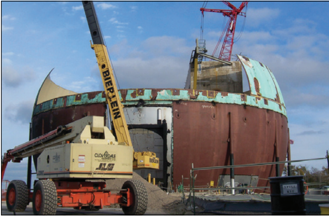
Demolition Activities at Big Rock Point Nuclear Power Plant Building debris is classified as Class A low-level radioactive waste
